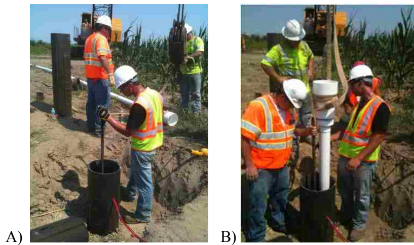
Figure 5.8 Process of Test Pile Concrete Placement. (A) Centerbar lowered into Test Pile. (B) PVC Tremme Lowered Around VWSGs.
