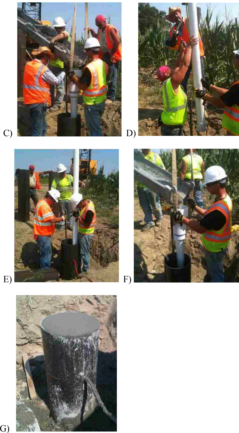
Figure 5.8 (cont.) Process of Test Pile Concrete Placement. (C) Begin Concrete Placement. (D) PVC Tremme Removed and Shortened with Sawzall. (E) PVC Tremme Re-lowered into Test Pile. (F) Resume Concrete Placement. (G) Concrete Placement Finished.
